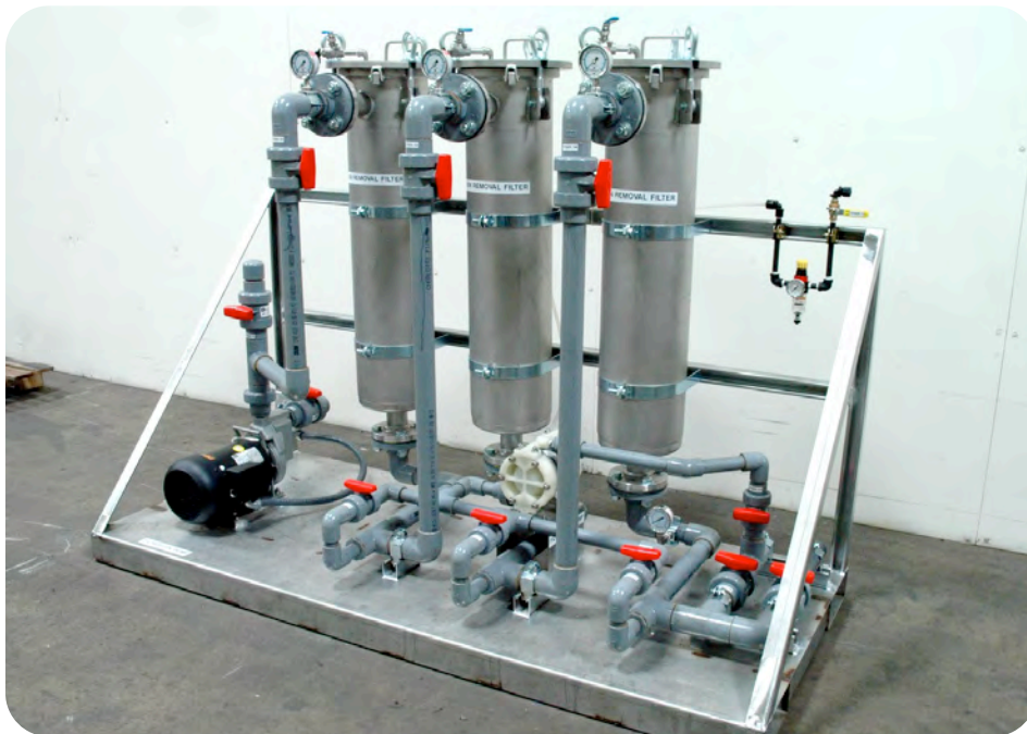
Graduated (Progressively Finer Filtration) Pickle Bath Filtration Skid
